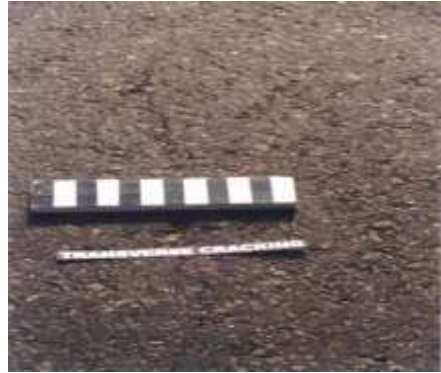
CRACKED ROAD (UNMODIFIED)
